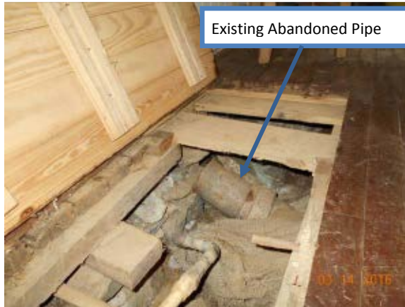
Figure 24: Crawl Space & Abandoned Pipe.
