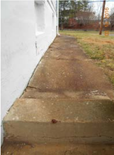
Figure 9: East Elevation Sidewalk Distress.
