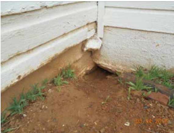
Figure 23: Undermined existing foundation wall.
