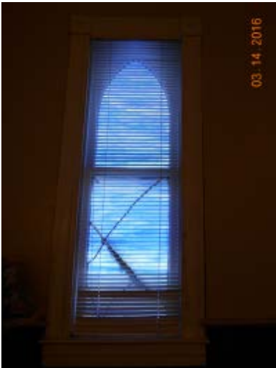
Figure 17: Cracked Window Panes.
