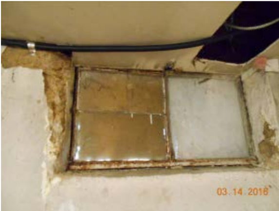
Figure 13: Moisture Distress @ Basement Window Surrounds.
