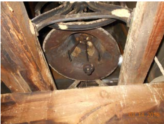
Figure 18: Bell Tower Framing Deterioration.
