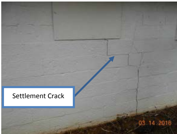
Figure 27: South Elevation Settlement Cracks.
