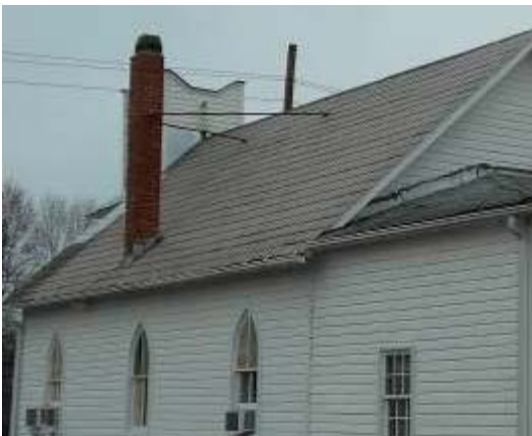
Figure 10: Deteriorated Mortar Joints @ Existing Chimney
