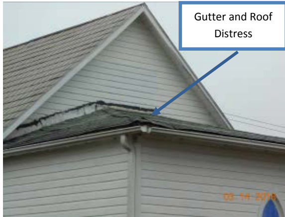
Figure 5: Roof and Gutter Distress.
