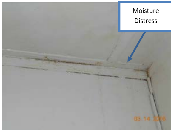
Figure 25: Moisture Distress @ Interior Walls.
