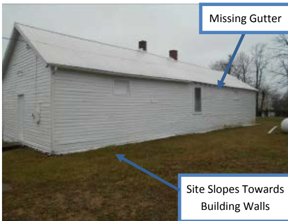
Figure 20: West Elevation Missing Gutter.
