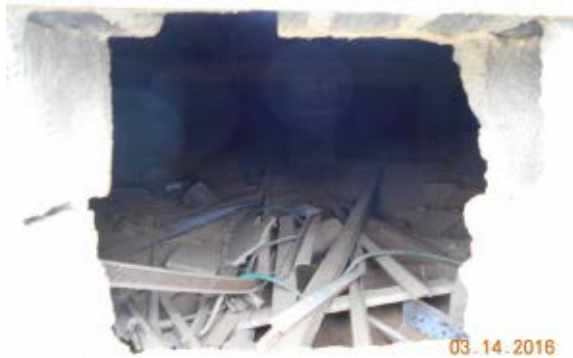
Figure 7: 1940's Foundation Unprotected Opening.
