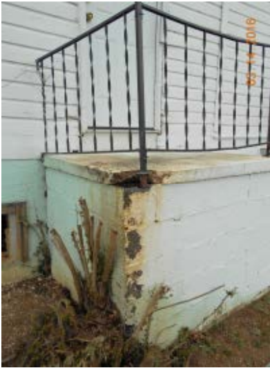
Figure 8: Spalled Railing Attachment.
