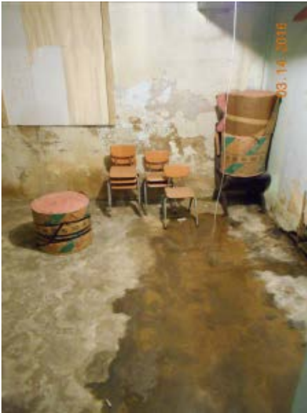
Figure 12: Standing Water and Moisture Staining @ Basement slab.
