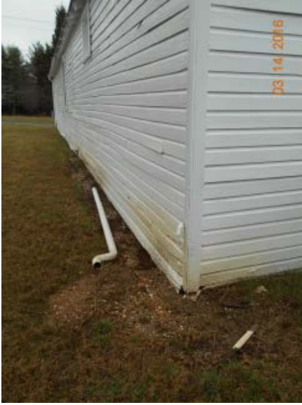
Figure 22: West Elevation Wall Displacement.
