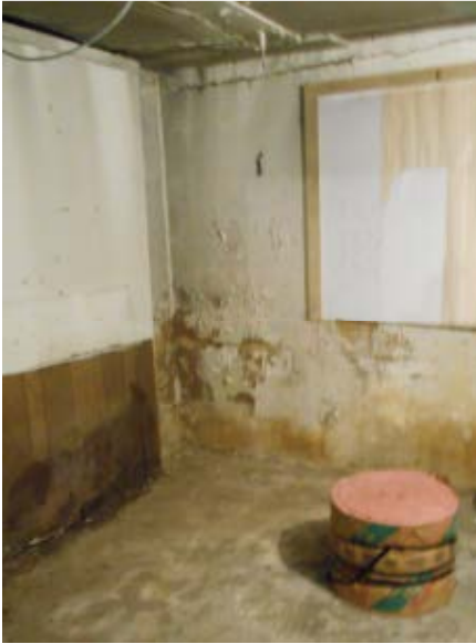
Figure 11: Rising Damp @ Interior Basement Walls.
