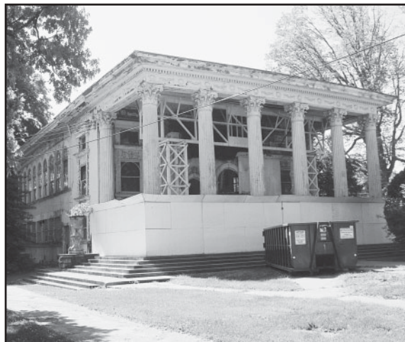
Due to exposure to the elements and years of neglect, the Classical Revival building which served as the gymnasium continues to deteriorate and out of safety concerns is closed to the public.
