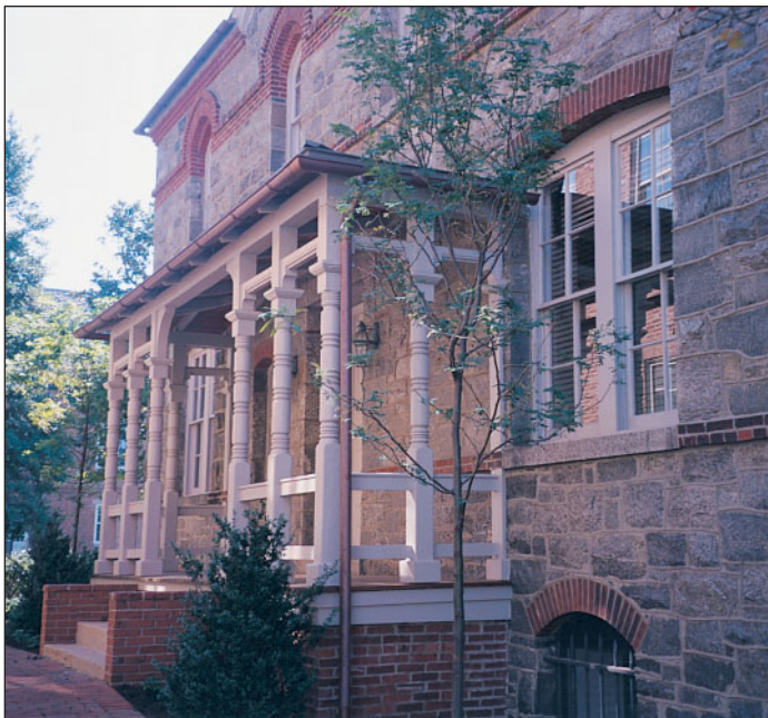
As part of the renovations being funded by the Save Maryland's Treasures program, the front porch of the 1881 Sheriff's House has been restored.
