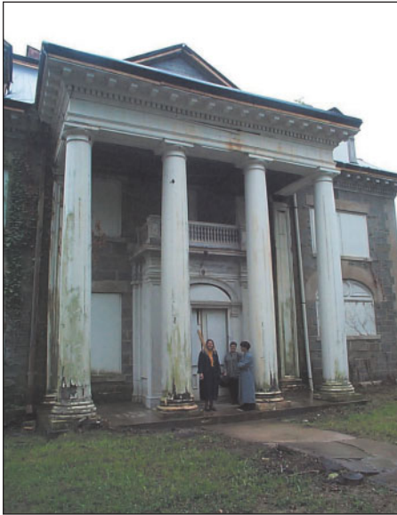
Preservation Maryland advocated for the historic Beaux-Arts campus of Cecil County's Tome School for Boys to be listed in the National Register of Historic Places and permanently protected by an easement held by the Maryland Historical Trust.
