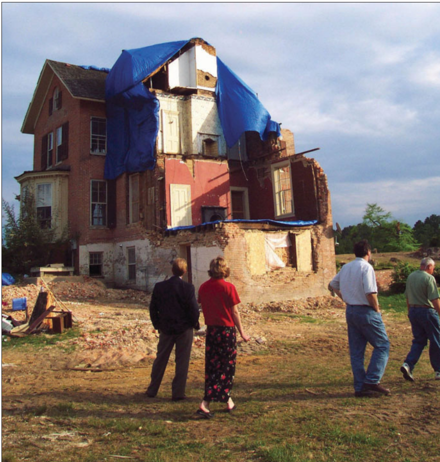
Preservation Maryland joined representatives from the Maryland Historical Trust and the Federal Emergency Management Agency to assess the F5 tornado damage to historic structures in LaPlata and assist with recommending technical and funding resources for stabilization and repair.
